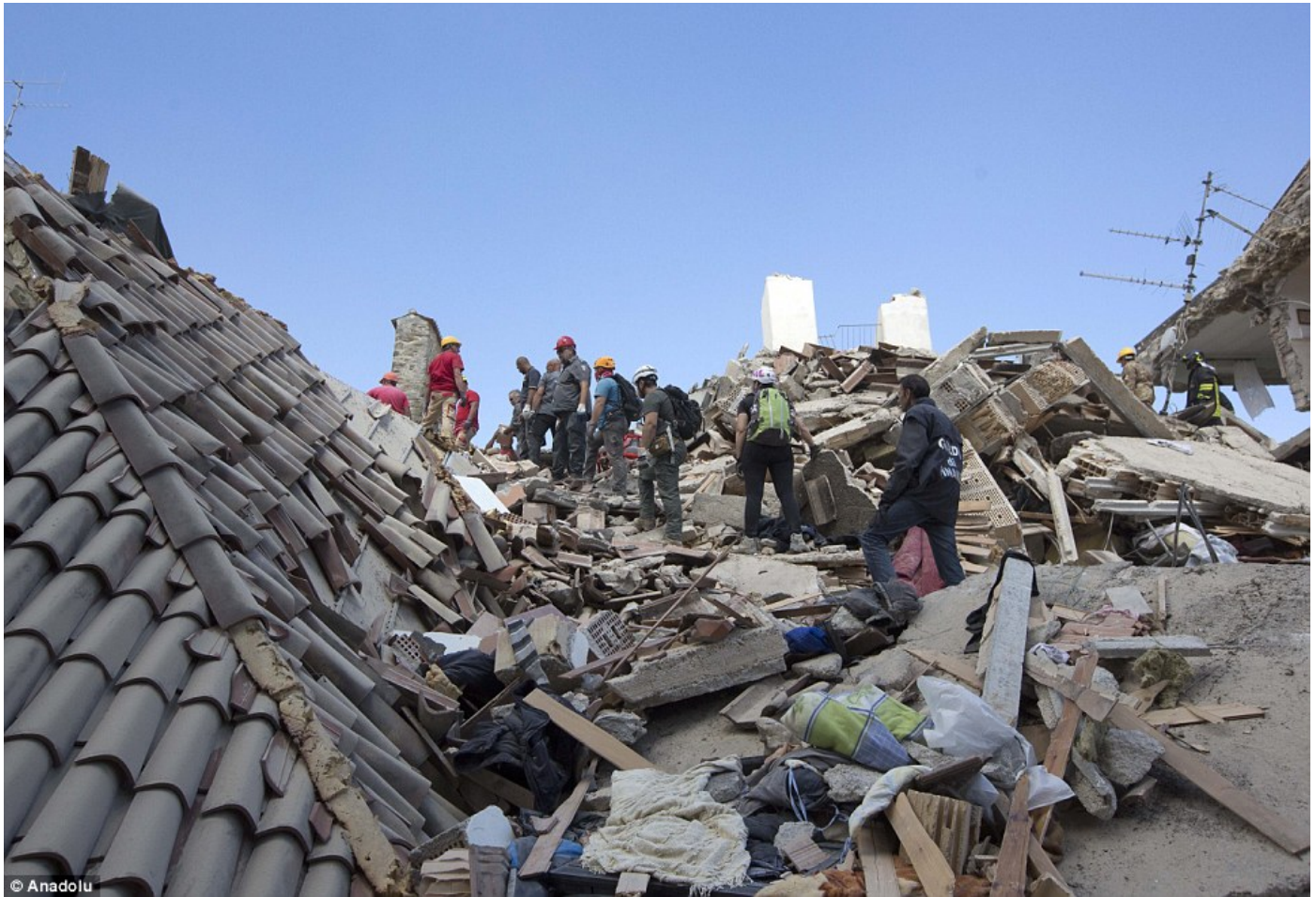
Rescuers scaled a roof in Amatrice as they continued their hunt for survivors
