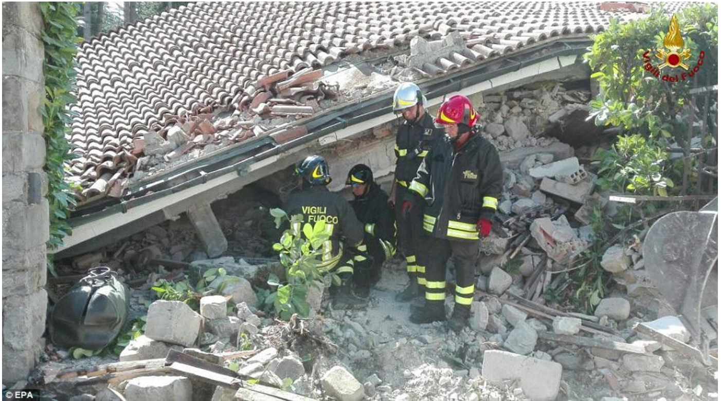
Signs of life: The Italian Fire brigade are seen working on a collapsed and damaged house in Amatrice which appears to have been reduced to a roof
