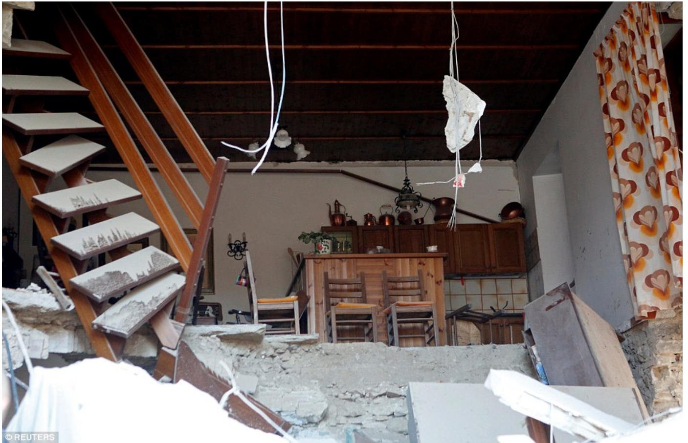
Contrast: The intact kitchen of this home lies completely undamaged - but exposed to the outside world after its wall fell away
